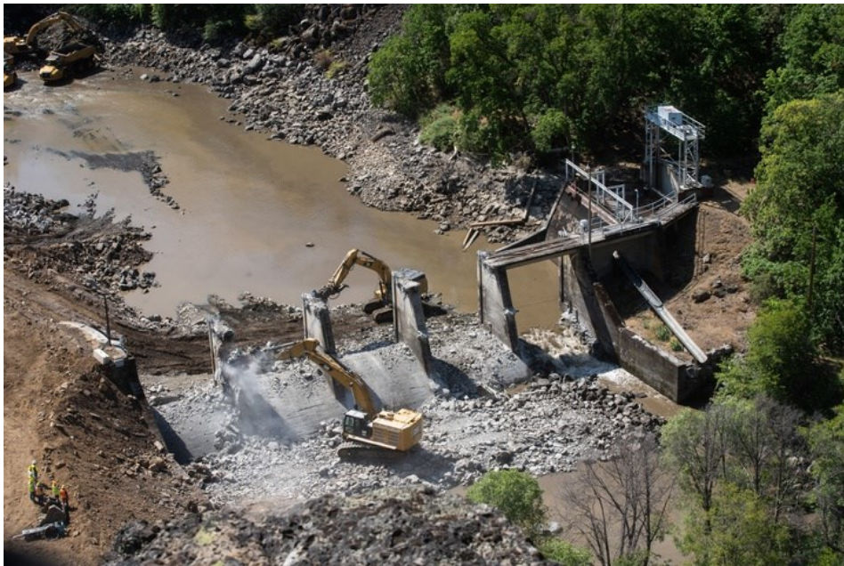
Kiewit crews deconstruct Copco No. 2, one of four Klamath River dams slated for removal. Photo by Shane
