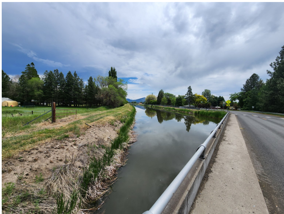
Photo of The a section of A Canal. This is one of several locations where short-term repairs have been made due to no water in 2021-related issues.
